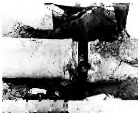
Photo 16. Eighteen-inch diameter steel water pipe, concrete lined. Joint opened by tension. Note recently repaired gas main in foreground. Los Angeles Department of Water and Power photo.
